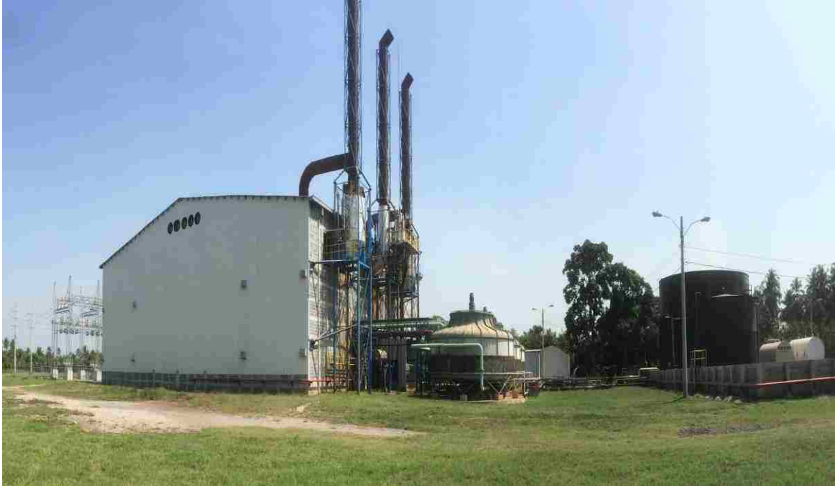
Figure 4.35. Panoramic view of Genosa Power Plant
