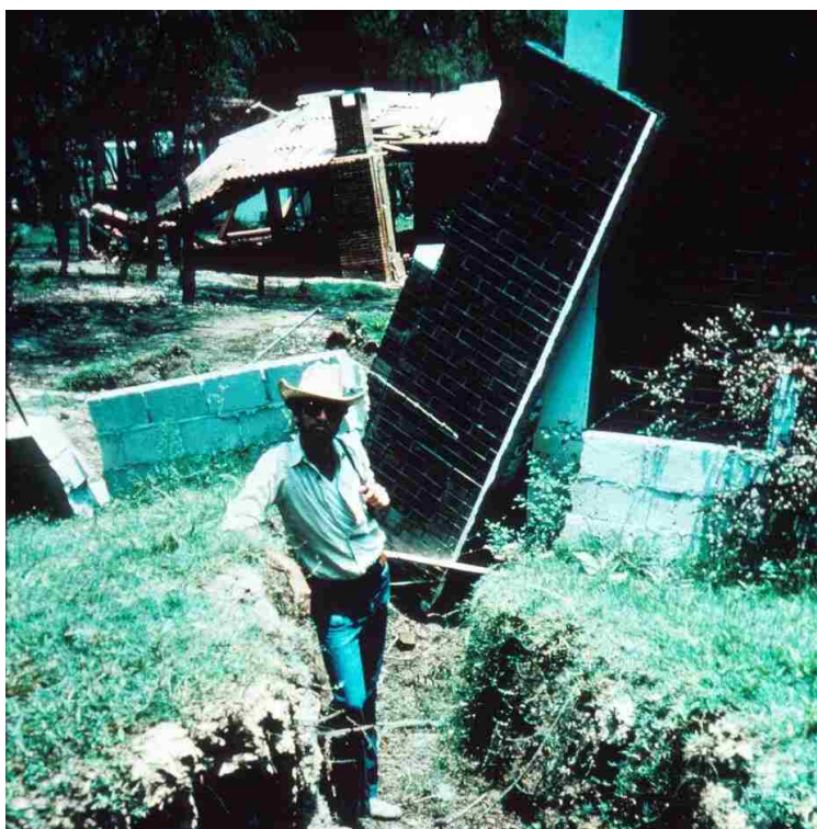
Figure 2.10. Cracks at Lake Amatitlan (Plafker, 1977)
